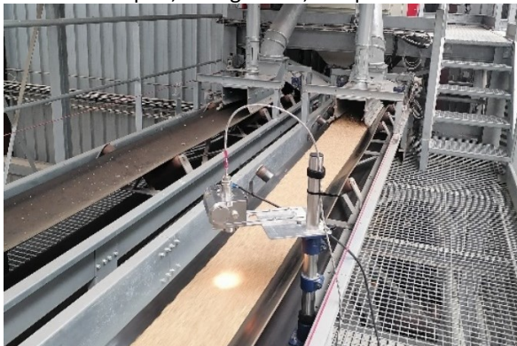
Figure 3 : Example of the installation of a distance sensor head on a test site (ARVALIS pilot site)
