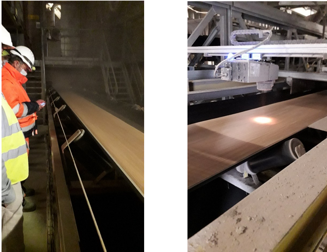
Figure 4: Examples of possible installation sites for distance head sensors in silos (on the left, on the frame of the conveyor belt with the addition of a support, on the right, on the existing support of another device).
